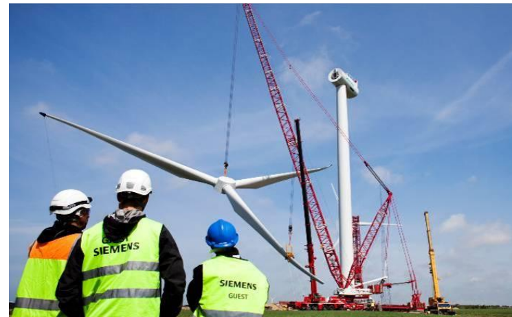
Prototype installation Høvsøre, Denmark
