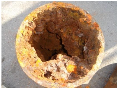
Before (Oct. 2011) 40% of pipe was clogged by scale and rust
