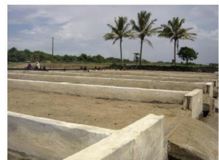
Sludge Drying Beds
