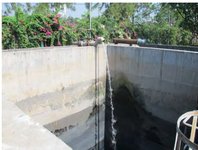
Figure 10: Wastewater receiving/balancing tank at CETP in IZ
