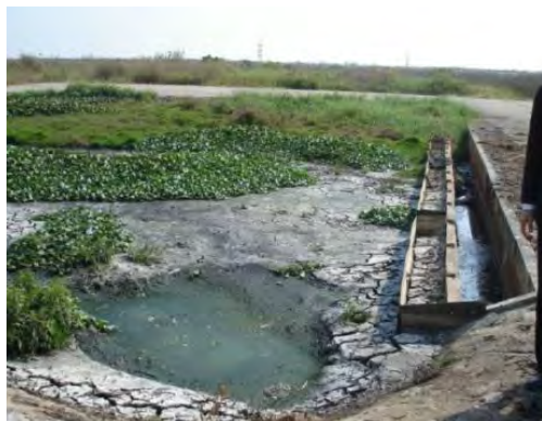
Sludge stabilization pond
