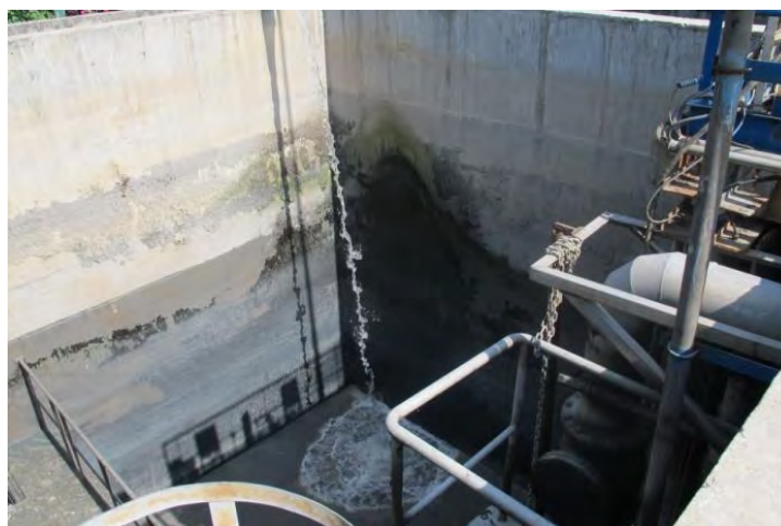
Figure 12: Incoming wastewater at CETP
