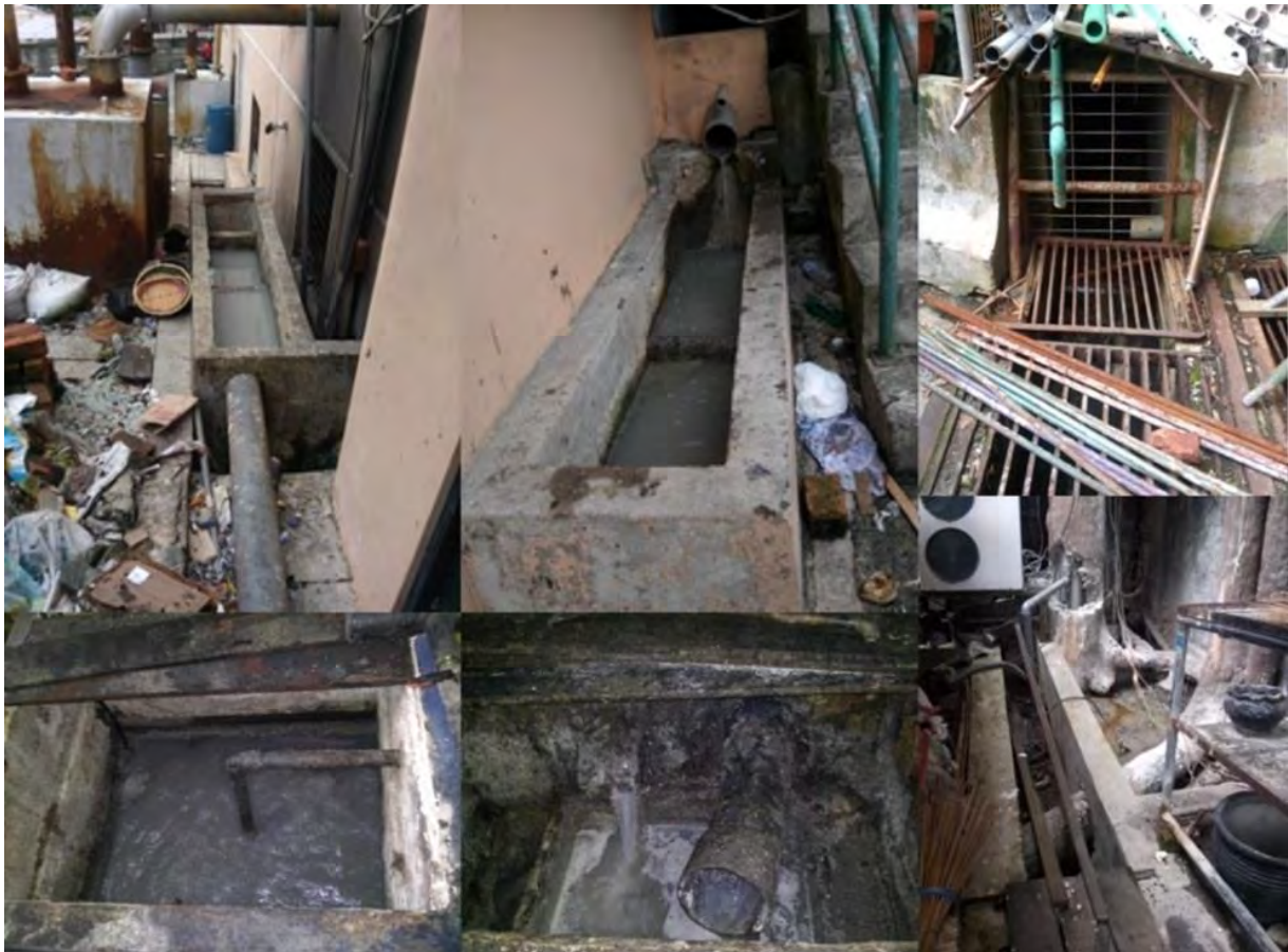
Figure 5: Wastewater treatment from kitchen and laundry of the Gran Senyur Hotel
