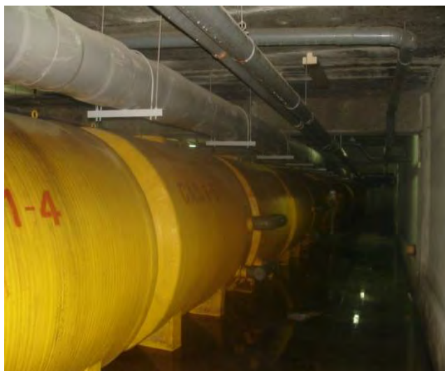
Figure 11: Packaged wastewater treatment station installed in a basement of a building
