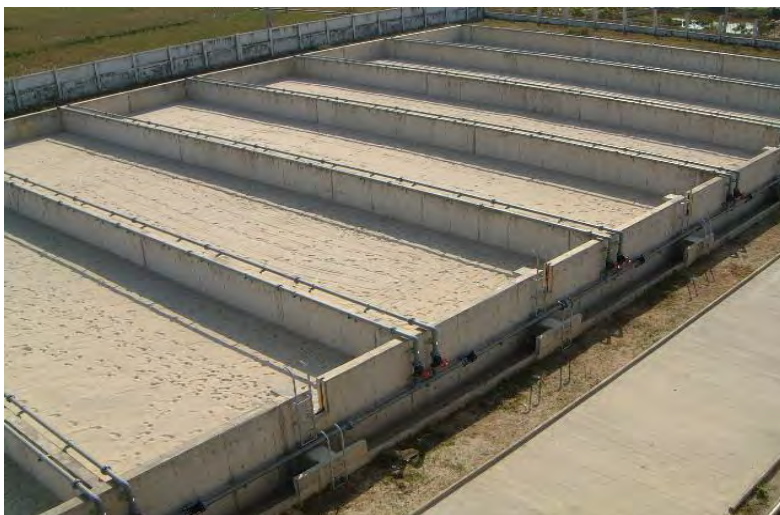
Figure 17: Sludge-drying beds are the most common technology for sludge dewatering at water treatment plants
