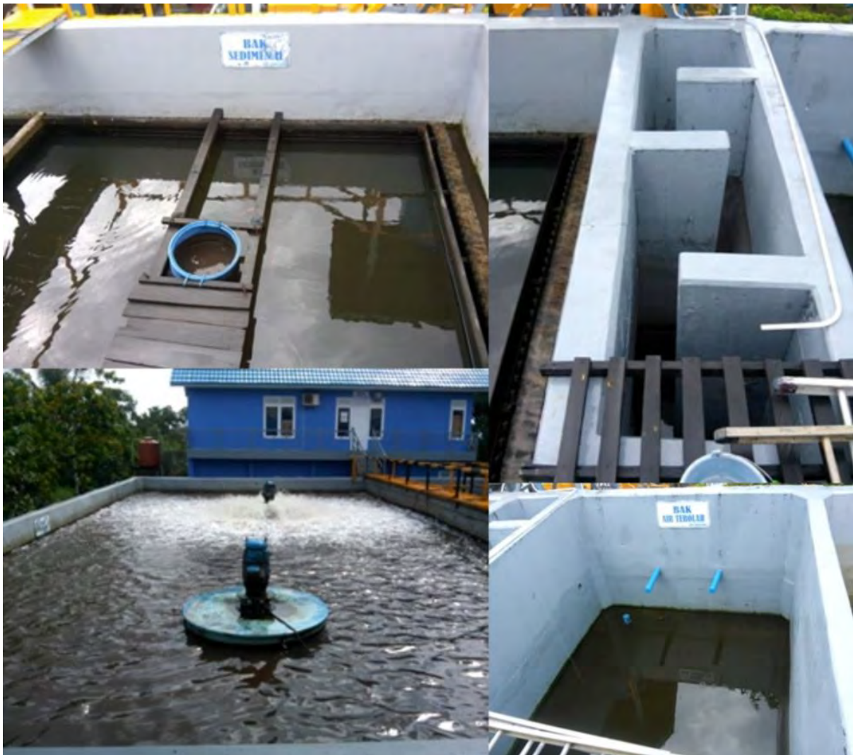
Figure 4: City Sludge Treatment-Balikpapan
