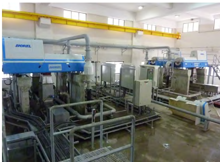
Figure 19: Mechanical sludge dewatering is an energy-consuming technology
