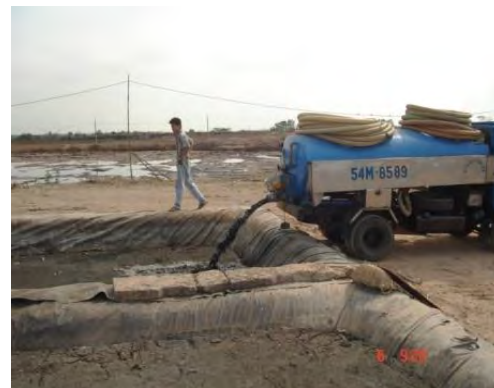
Sludge drying and composting fecal sludge treatment technologies applied in Viet Nameese cities
