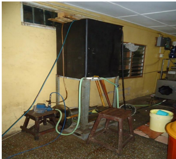
Photo 8: Picture of water storage container with an electric pump
