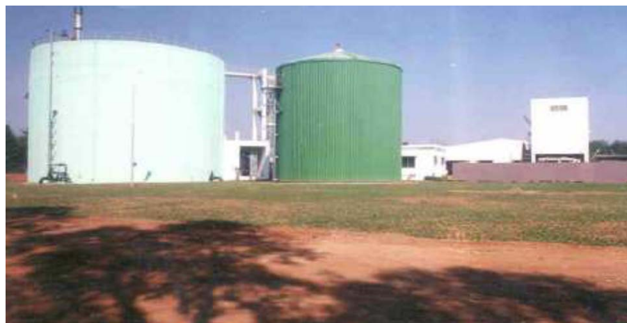
3000 cum biomethanation project for solid waste at Slaughterhouse in Andhra Pradesh
