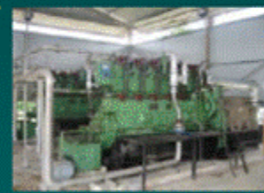
Fuel for CHP
